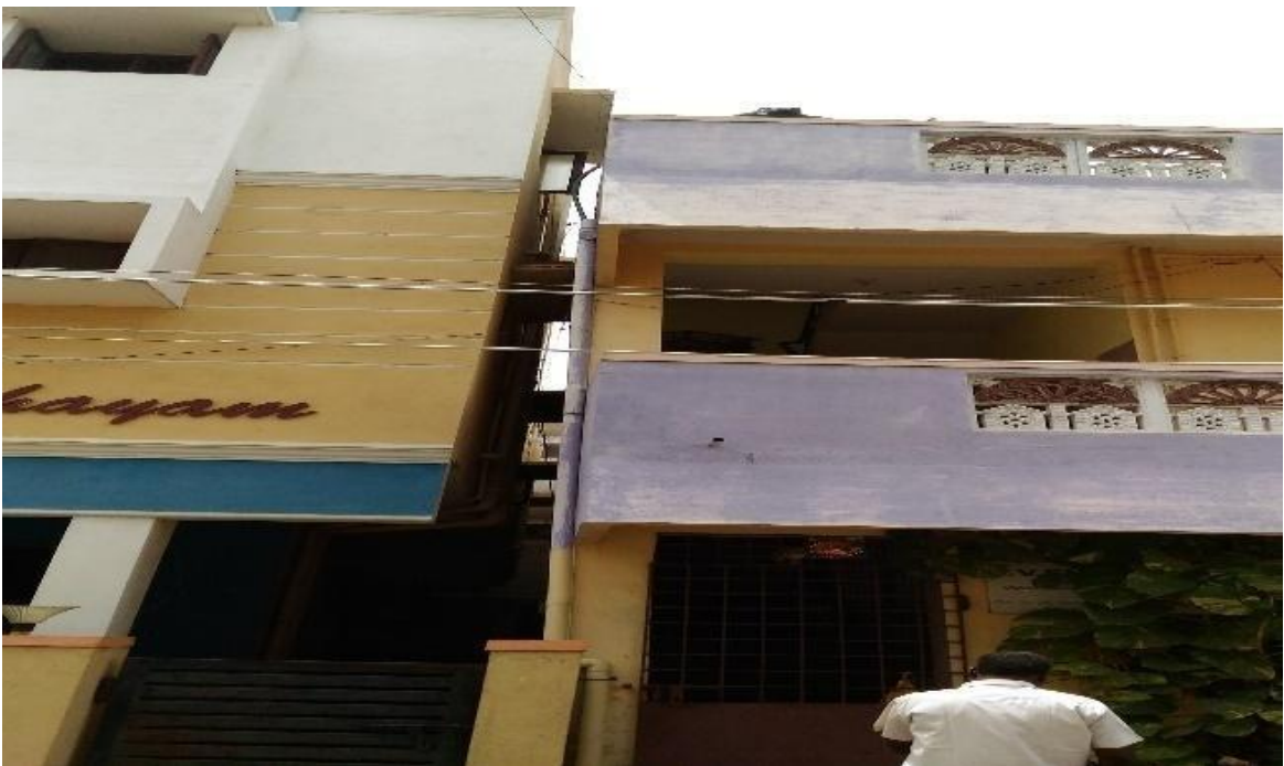
Building tilting on western side of the plot. -2
