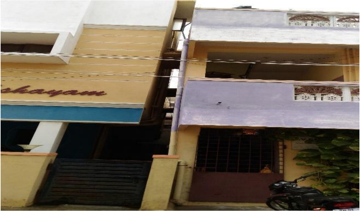
Building tilting on western side of the plot. -1
